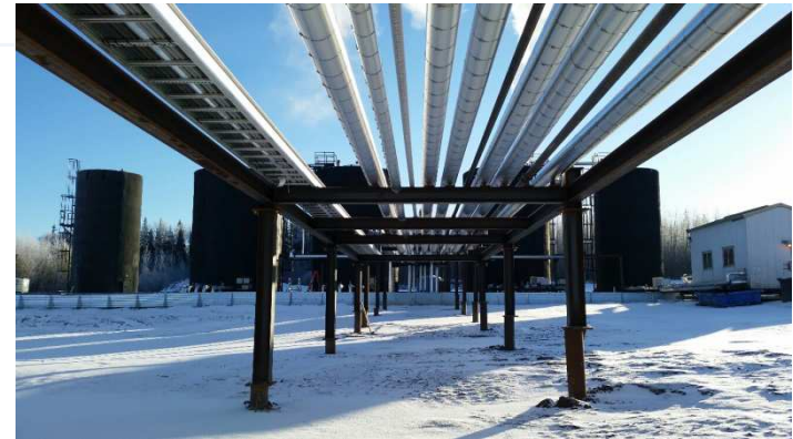
Pipe rack tank farm
