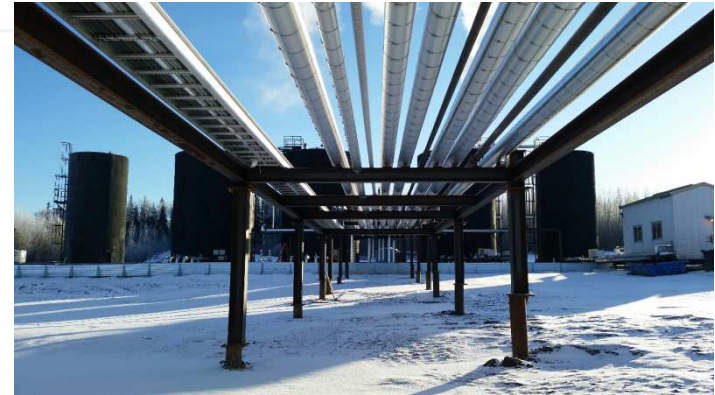
Pipe rack tank farm
